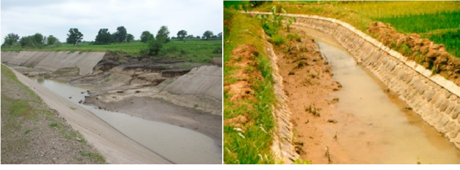
Fig. 1. Bank deterioration (left) and siltation (right) in irrigation canals.
